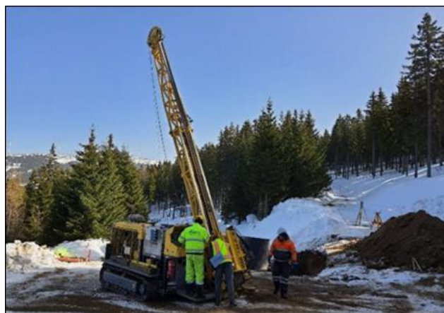
Figure 7-6: GEOPS rig drilling hole P18-09 as part of the 2021 drilling program Source: European Lithium/DRA
